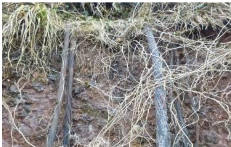
Cables uncovered by landslide
